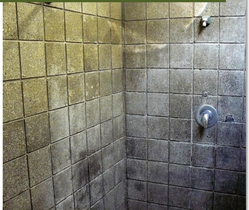
Example of mineral deposit, efflorescence and soap scum build-up.
